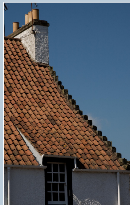
Clay pantiles and a 'catslide' dormer on a 17th-century house, Falkland, Fife. The roof sweeps up a little towards the eaves. © N. Haynes.
